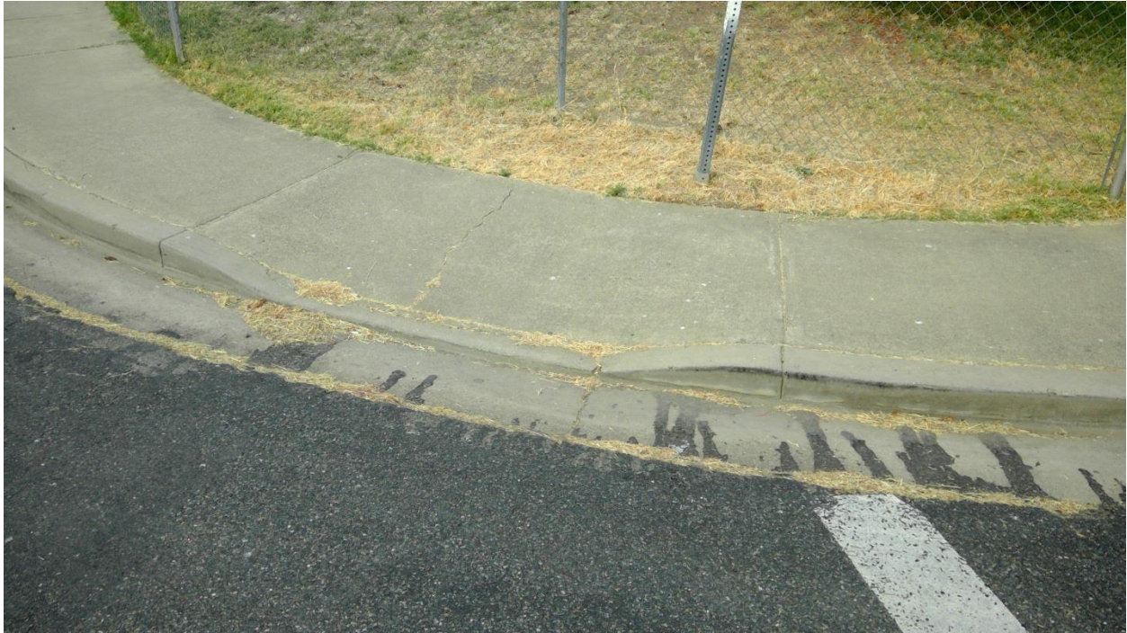
Figure 5: Example of ADA non-compliant curb ramp (Data entry #181)
